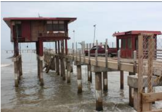
Pier damaged by Ike
